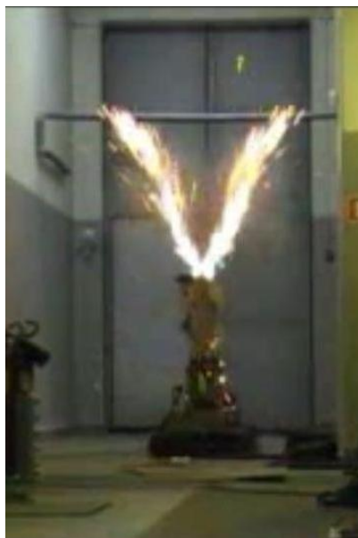
Fig. 2. The proper short circuit current switching off of an expected value of 50 kA [the frame of the film recorded by P. Andrzejewski]
