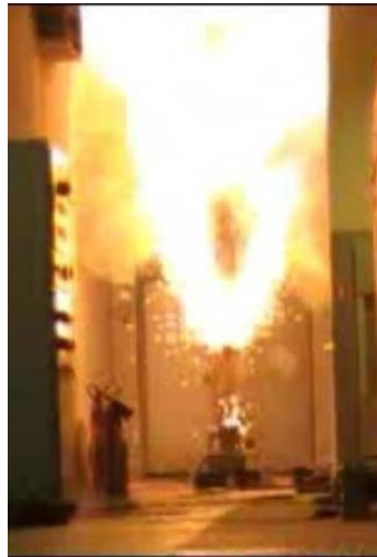
Fig. 4. View of a malfunctioned circuit switching off [frames of the film recorded by P. Andrzejewski]
