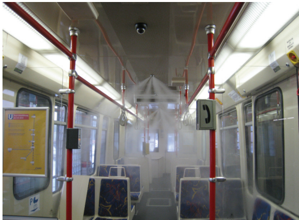
Fig. 9. Sectional activation of a high pressure water mist system in a passenger vehicle (train type „German U-Bahn”)
