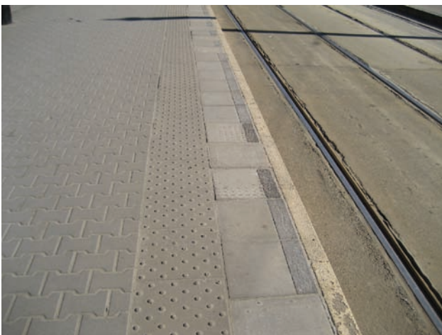
Fig. 10. Example of incorrect maintenance of platform edge [Photo J. Poliński]
