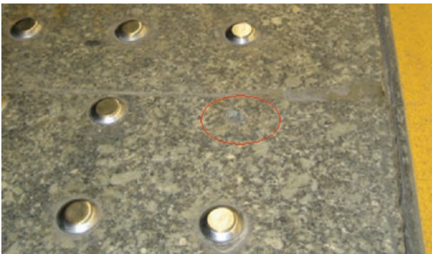
Fig. 8. Torn off truncated dome from the warning strip [Photo J. Poliński]
