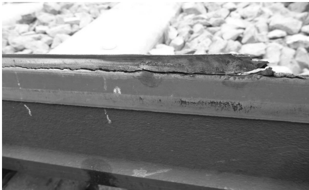
Fig. 4. Crack propagating near spallings of material of the switch rail [photo. M. Czarnecki]
