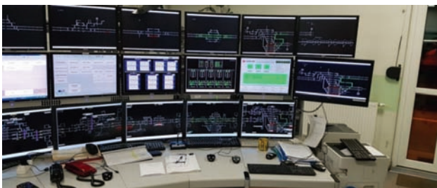
Fig. 4. Local control centre equipped with RBC [authors' own source]
