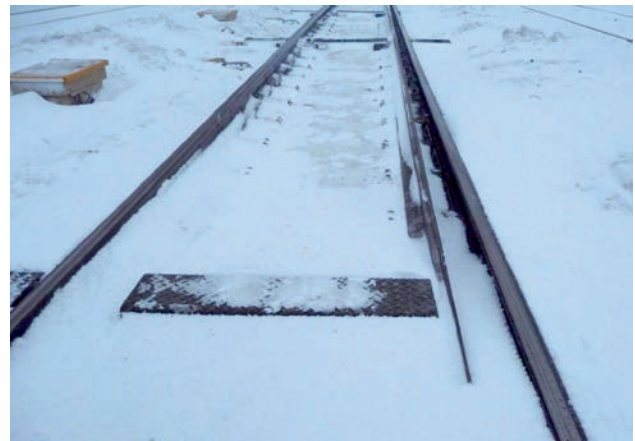
Fig. 3. Inefficient melting out the snow in the switch blade edge zone during intense snowfalls. The visible irregularity of melting out the snow along the stock-rail [PKP PLK January 201]
