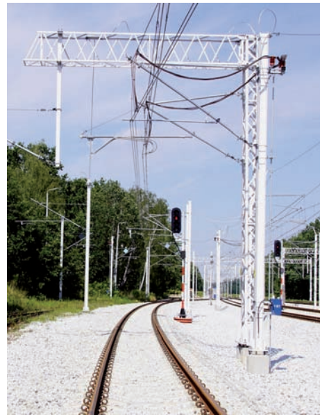
Fig. 1. Insulated six-post tension span with an isolating switch; YC120-2CS150 type overhead contact line, Łódź Żabieniec, 2021 [photo taken by D. Dratwa]
