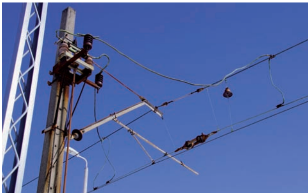
Fig. 6. Suspension at the air gap, with insulators in the catenary wire and contact wire; original ceramic section insulator and a dropper insulated by a ceramic single-shed strain insulator are preserved; sKB70-C type overhead contact line, Czachówek Południowy, 2018 [photo taken by D. Dratwa]
