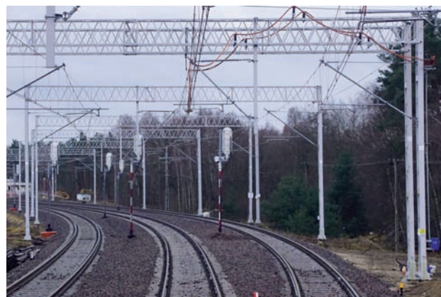
Fig. 15. Section insulator at disconnector No. 17 in the location of isolated tension span of an isolating switch No. 3, middle anchorage at the insulation, Chociszew 2021 [photo taken by D. Dratwa]
