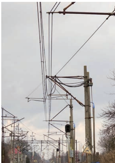
Fig. 9. Shortened isolated six-post tension span, YC150-2C150 type overhead contact line, Zielonczyn, 2016 [photo taken by D. Dratwa]
