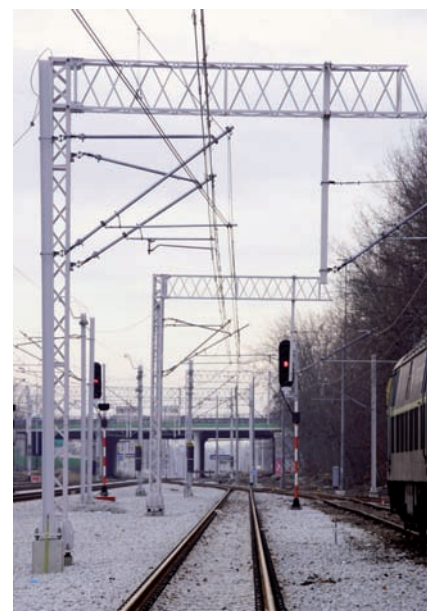
Fig. 2. Insulated six-post tension span without an isolating switch or sectional disconnecter; YC120-2CS150 type overhead contact line, Łódź Żabieniec, 2021 [photo taken by D. Dratwa]
