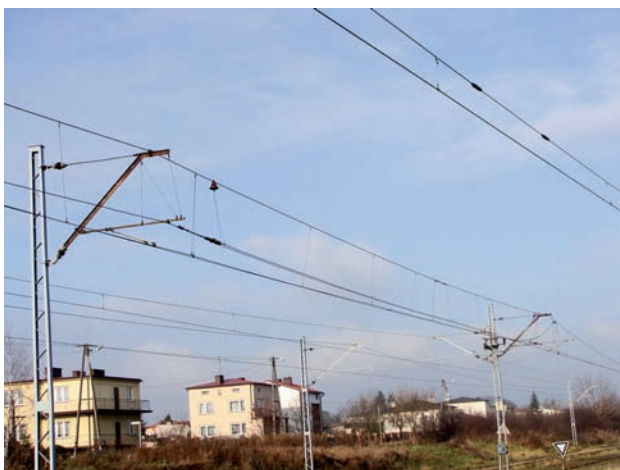
Fig. 7. Air gap with insulated catenary wire in the middle of the passage; C120-2C type overhead contact line, Głowno, 2010 [photo taken by D. Dratwa]
