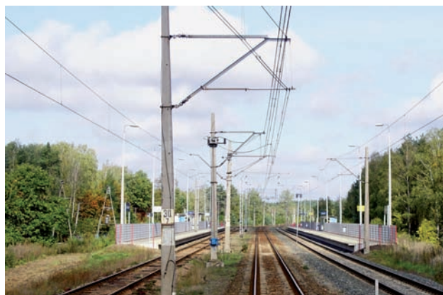
Fig. 13. Isolated tension span of an isolating switch No. 1 on a straight track in Chociszew before station reconstruction, 2019 [photo taken by D. Dratwa]
