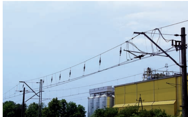
Fig. 8. Air gap with insulated catenary wire at one of the suspensions (on the right) and insulated droppers. Ceramic divider insulators from the time of electrification are preserved in the contact wires; droppers insulated with ceramic double-shed strain insulators. YC120-2C type overhead contact line, no Y auxiliary wires at gap suspensions, Żerków, 2018 [photo taken by D. Dratwa]
