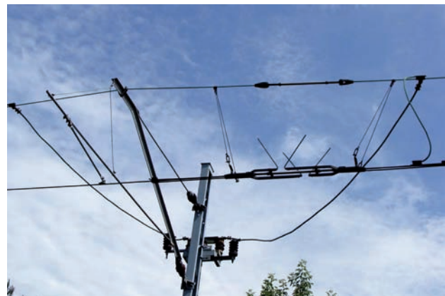
Fig. 3. Suspension with a section insulator made of plastic and an isolating switch; sKB70-C type overhead contact line, Głowno, 2011 [photo taken by D. Dratwa]
