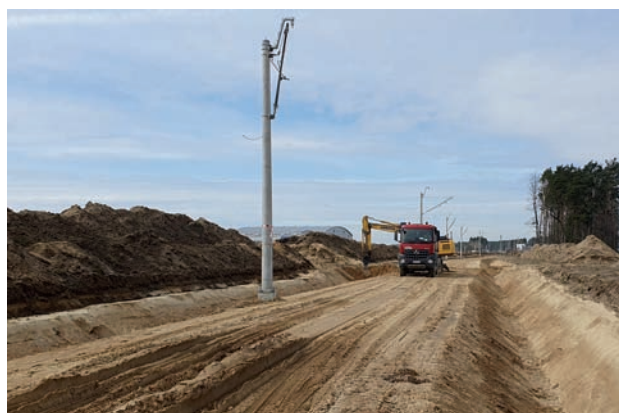
Fig. 15. Construction of railway line to Rzeszów Jasionka Airport (1 April 2023) [photo: P. Hamarnik / PLK]
