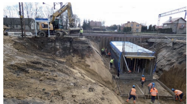
Fig. 20. Construction of a tunnel at Żurawica Station on LK 91 (1 April 2023) [photo: A. Mirek / PLK]
