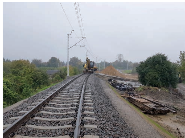
Fig. 9. Construction of the railway connector (LK 588) in Lublin [photo by M. Tyburk/PLK]
