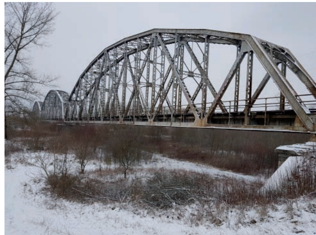
Fig. 21. The LK 68 before reconditioning and the bridge over the San River at Kępa Rzeczycka (Kępa – Pilchów section) [photo by PLK]
