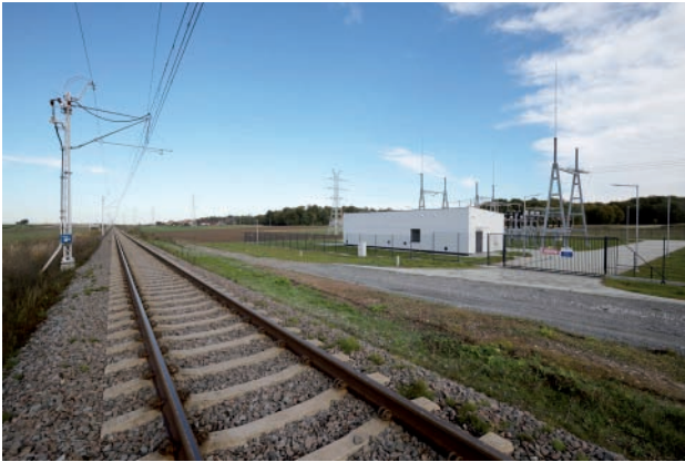
Fig. 12. Rzeczyca traction substation (6 October 2020) [photo by L. Brylowski/PLK]
