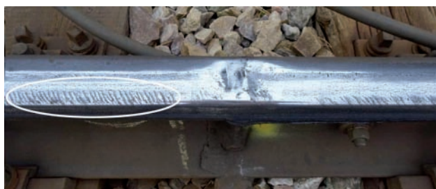
Fig. 2. Head checks of varying severity in the immediate vicinity of the welded joint [photo by I. Mikłaszewicz]
