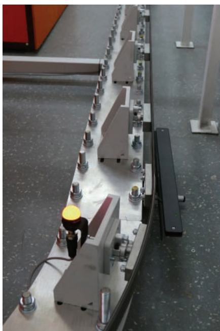
Fig. 8. Light signal (red light) and RFID antenna (right) [photo by J. Moczarski]
