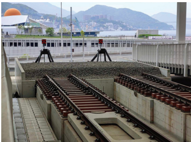
Fig. 9. Fixed (non-sliding) track end device at Nagasaki Station, Japan [photo by M. Peryt]
