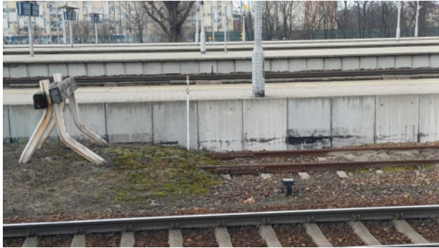
Fig. 7. Example of a track end device structure at Warszawa Wschodnia Station [photo by W. Kowalczyk]
