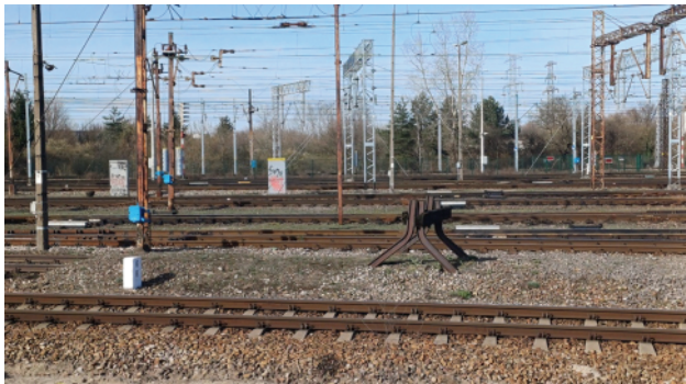
Fig. 8. Fixed (non-sliding) buffer stops – structures according to the BN-79 9310-06 standard at Warszawa Grochów Station [photo: D. Kowalczyk]
